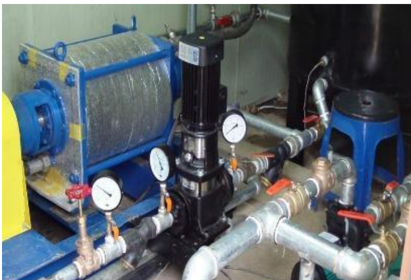
Figure 3 - Climate control systems
