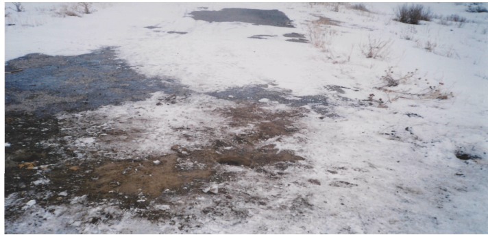
Figure 9 - Drilled road construction in the middle of the road, in the middle of traffic path and edge
